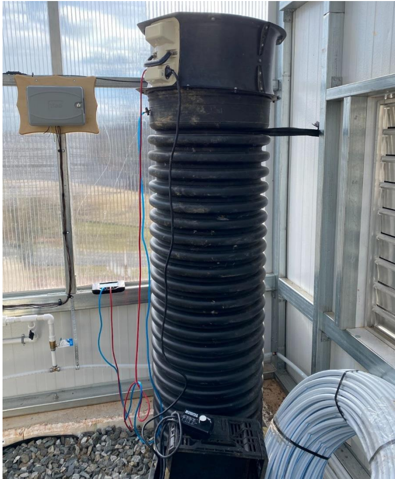
Figure 8: Image of Calibrated Fan setup for flow measurements of the GAHT
